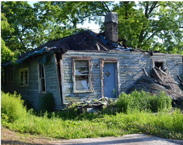
Dilapidated house in Titusville.
