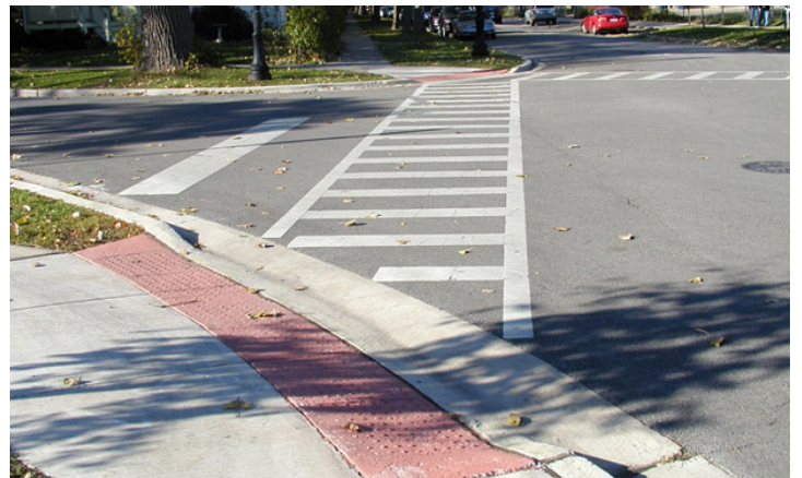
ADA curb ramp and crosswalk at an intersection (Source: Lee Engineering, LLC.)
