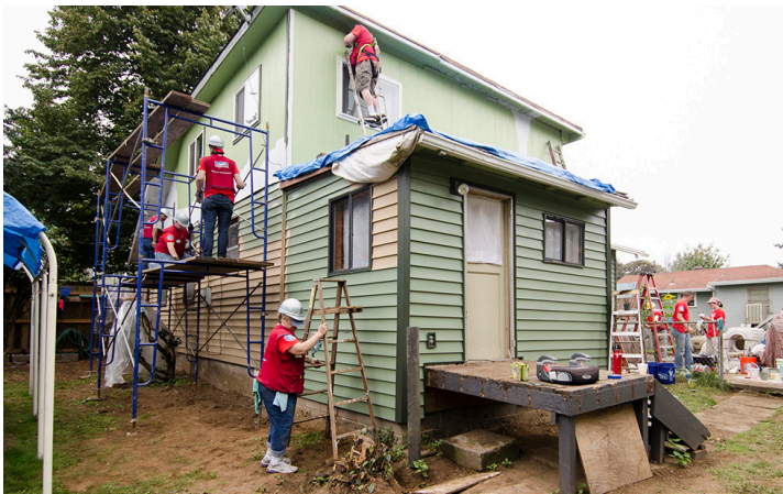
Rock the Block volunteers repairing a house (Source: Habitat for Humanity Portland/Metro East)
