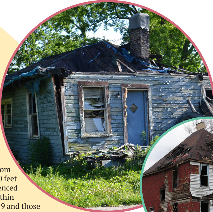
Above and Right: Dilapidated houses
